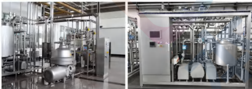
Pre-pasteurization and cream separator system
