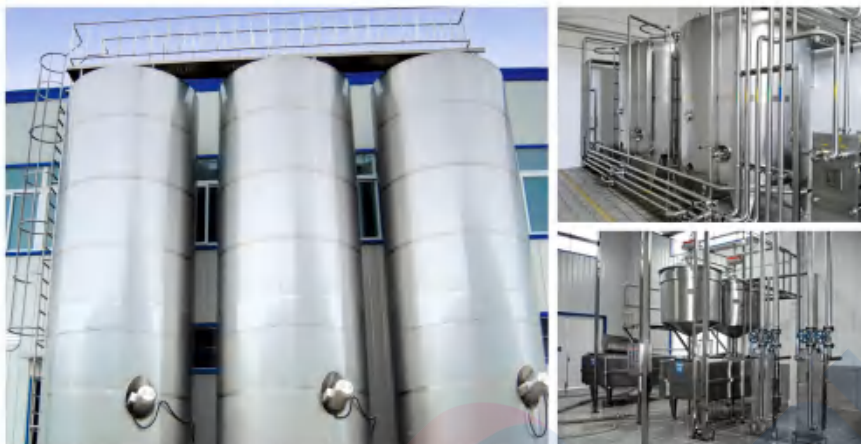
Milk receive and storage system
